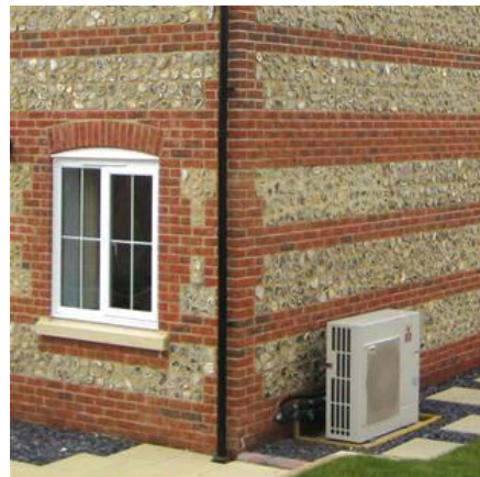
Air Source Heat Pump
